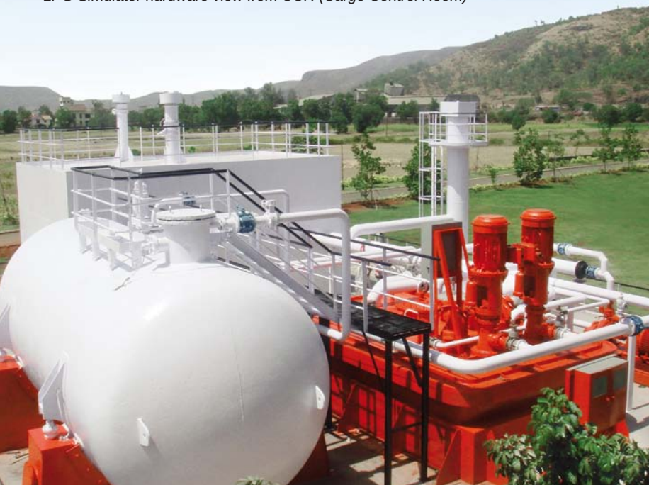
LPG Simulator hardware view from CCR (Cargo Control Room)
